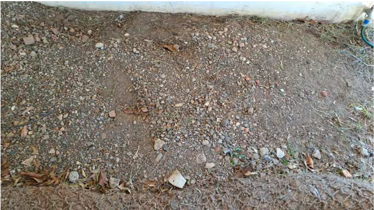
Image 6.11.2 View of shallow filling observed in garden bed, along the southern wall of the house
