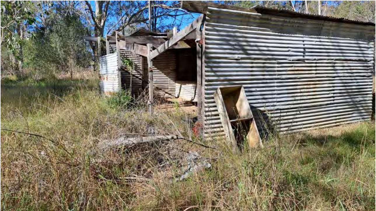
Image 6.2.3 View of metal shed (shed 2) with damaged roofing, facing west
