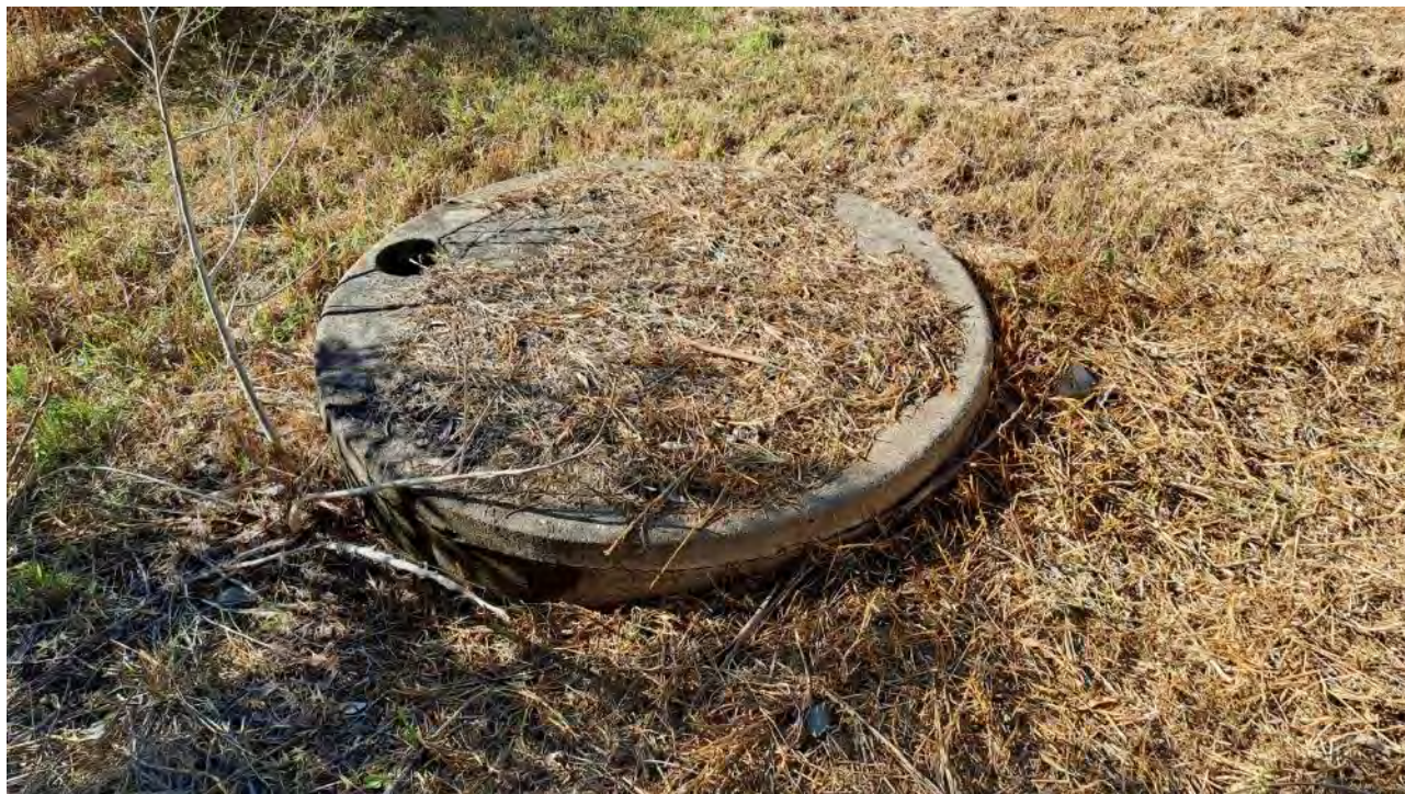
Image 6.8.1 View of septic system located to the north of the house
