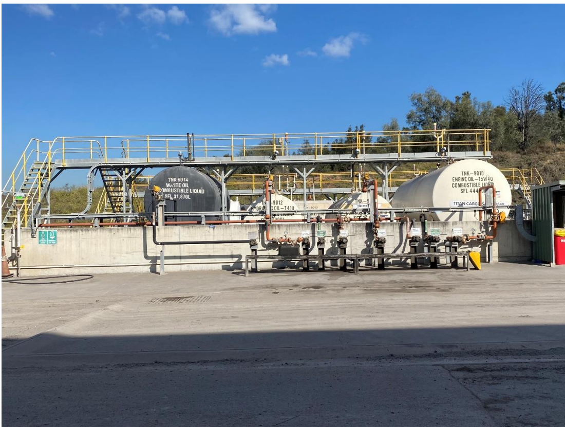
Photograph F.77 Oil storage
