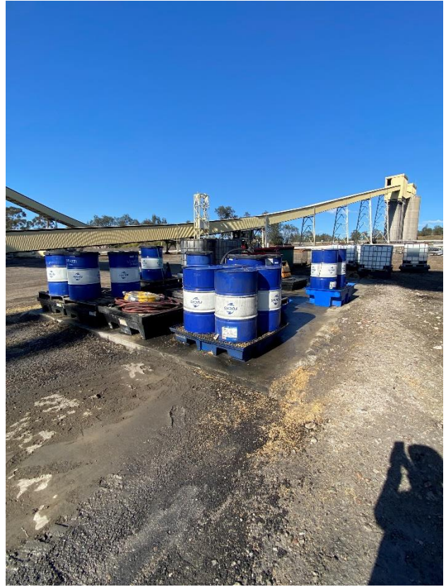
Photograph F.34 Hydrocarbon storage
