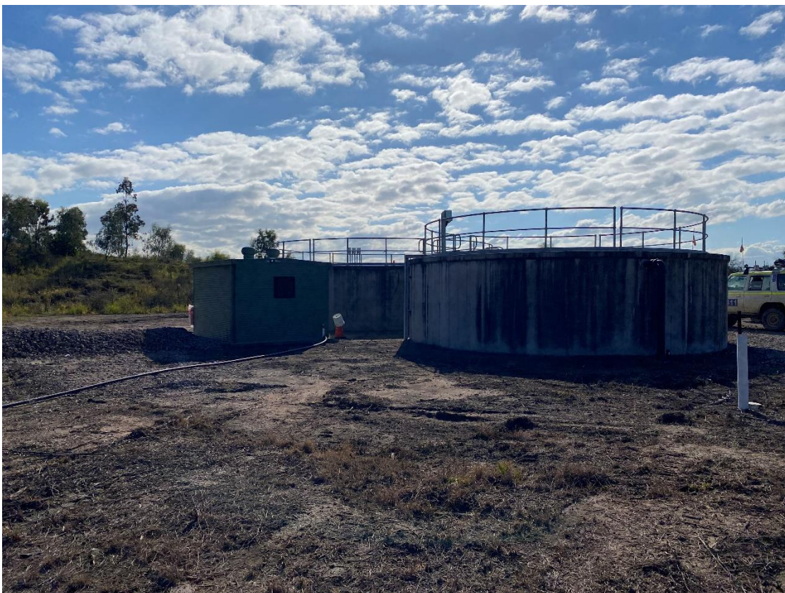
Photograph F.57 Sewage treatment system
