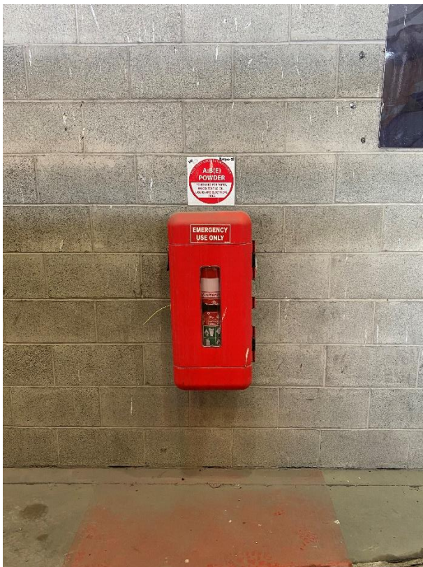
Photograph F.60 Fire extinguisher
