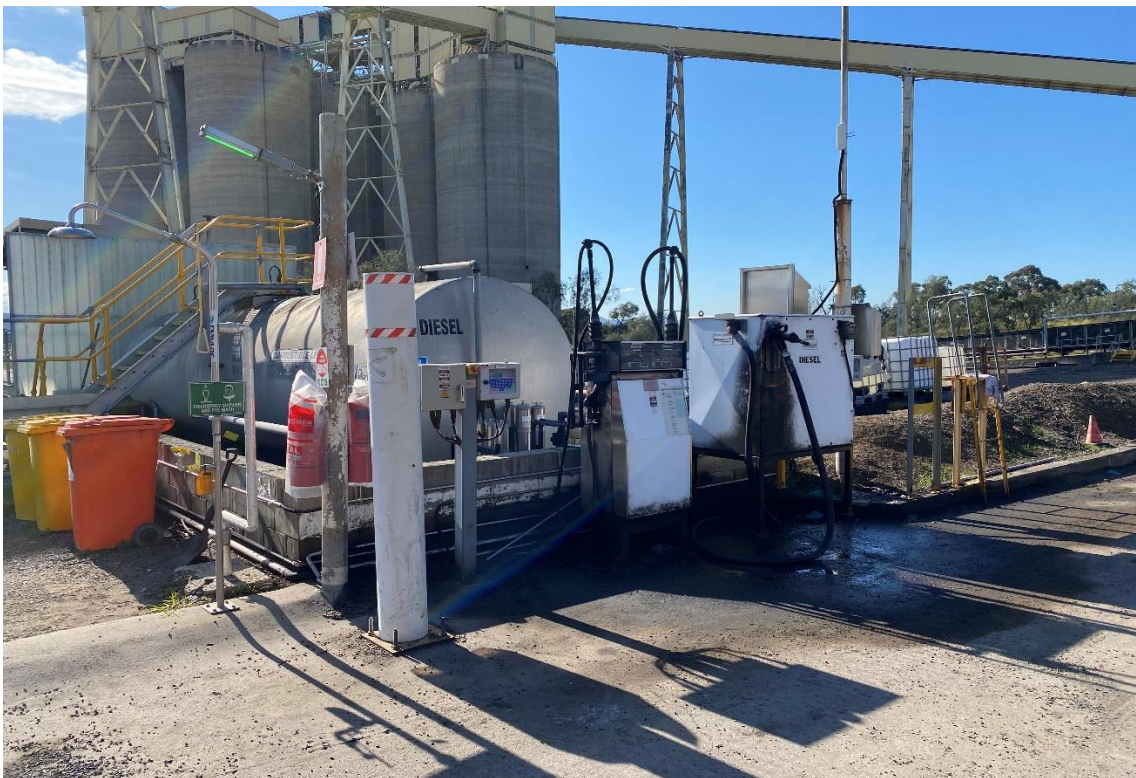
Photograph F.51 Diesel storage and pump
