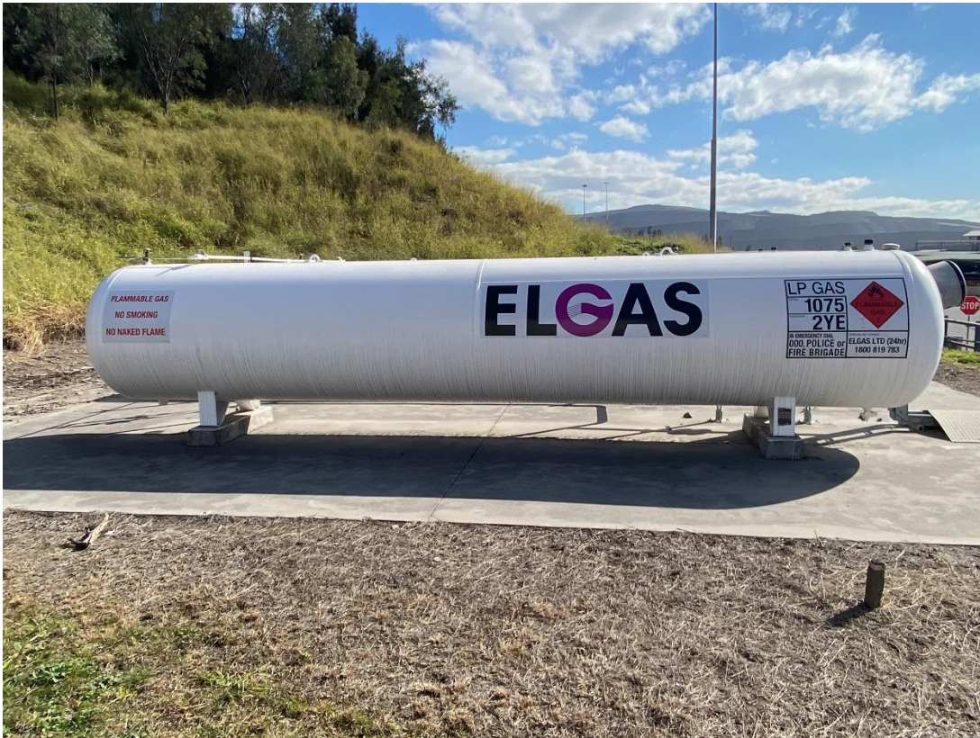
Photograph F.80 Gas storage
