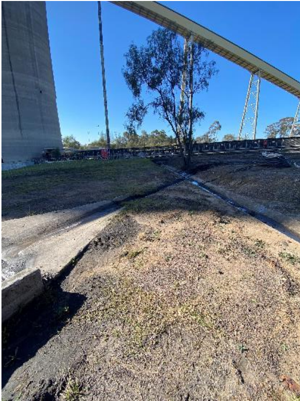
Photograph F.44 CHPP water runoff
