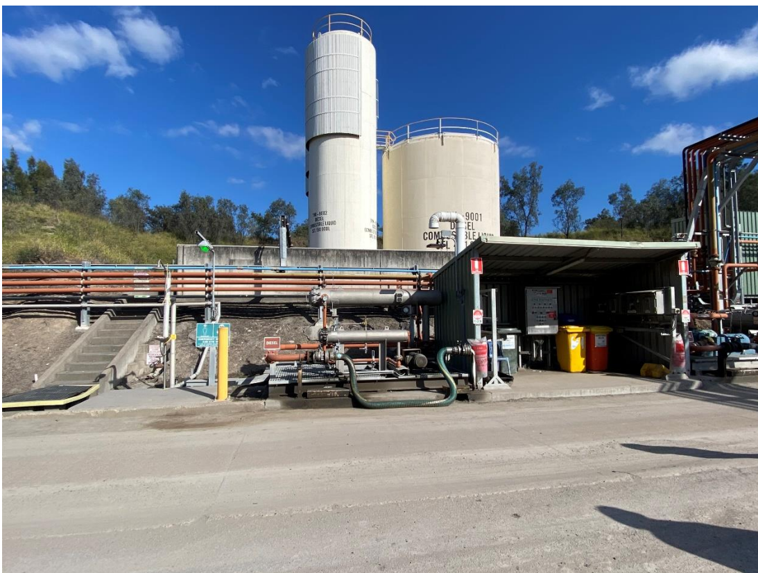
Photograph F.79 Diesel storage
