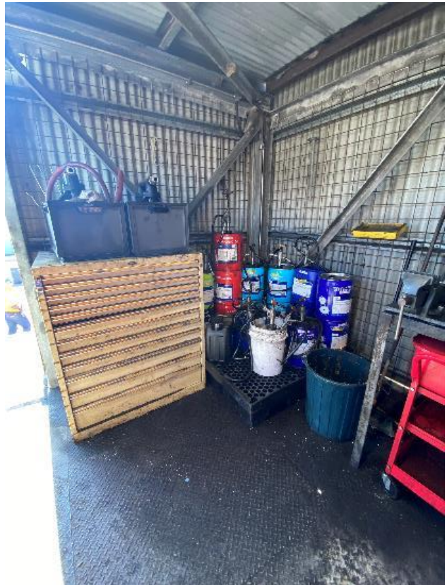
Photograph F.39 Hydrocarbon storage
