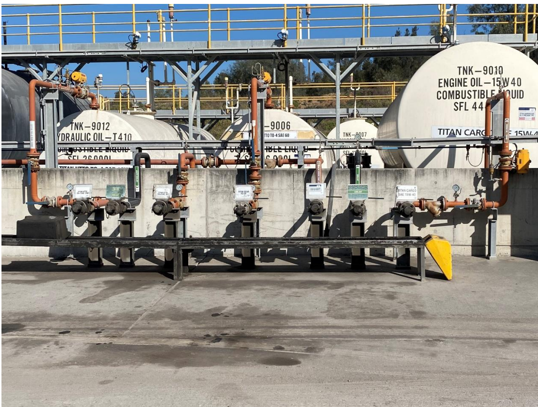
Photograph F.75 Oil storage
