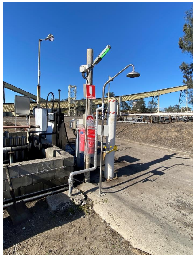
Photograph F.47 Emergency shower and eye wash
