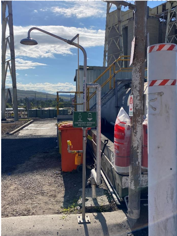
Photograph F.52 Emergency shower and eye wash
