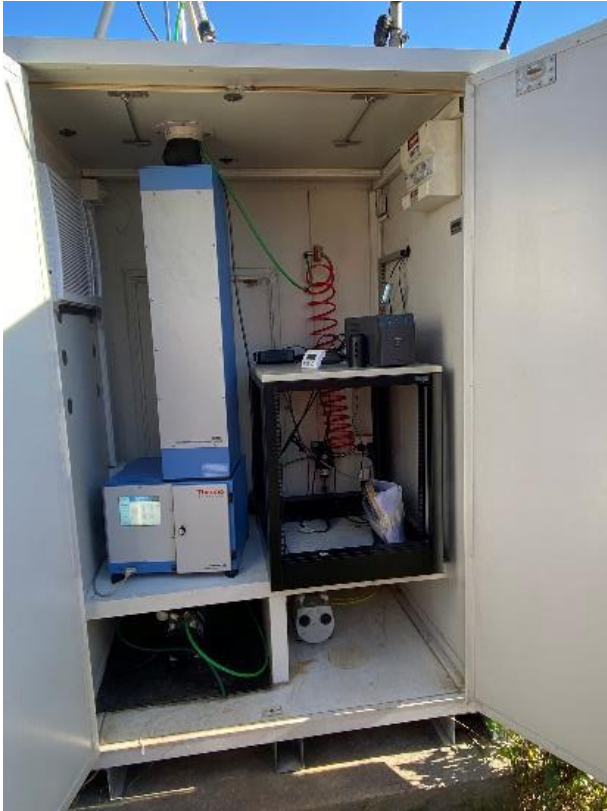
Photograph F.18 Air quality monitoring station
