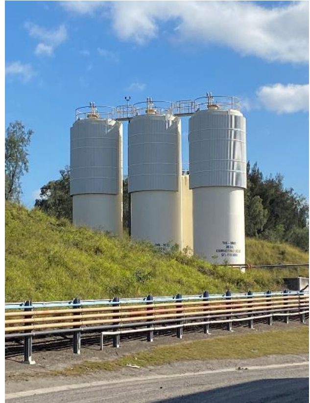
Photograph F.74 Diesel storage
