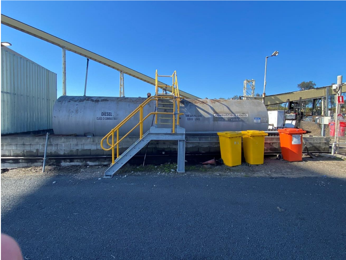
Photograph F.50 Diesel storage
