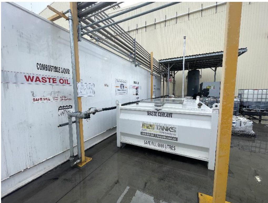
PHOTO 8 Waste oil and waste coolant storage
