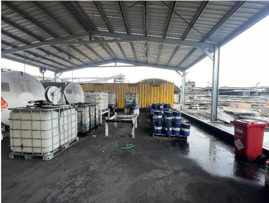
PHOTO 5 Chemical Storage area
