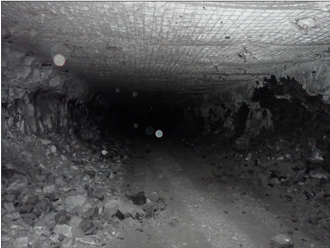
Figure 4: Rib deformation in 205 Panel X HDG, 9CT at 200m DOC.
