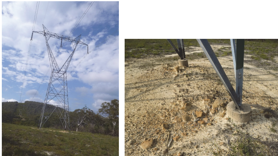
Fig. 6.3 330 kV transmission tower
