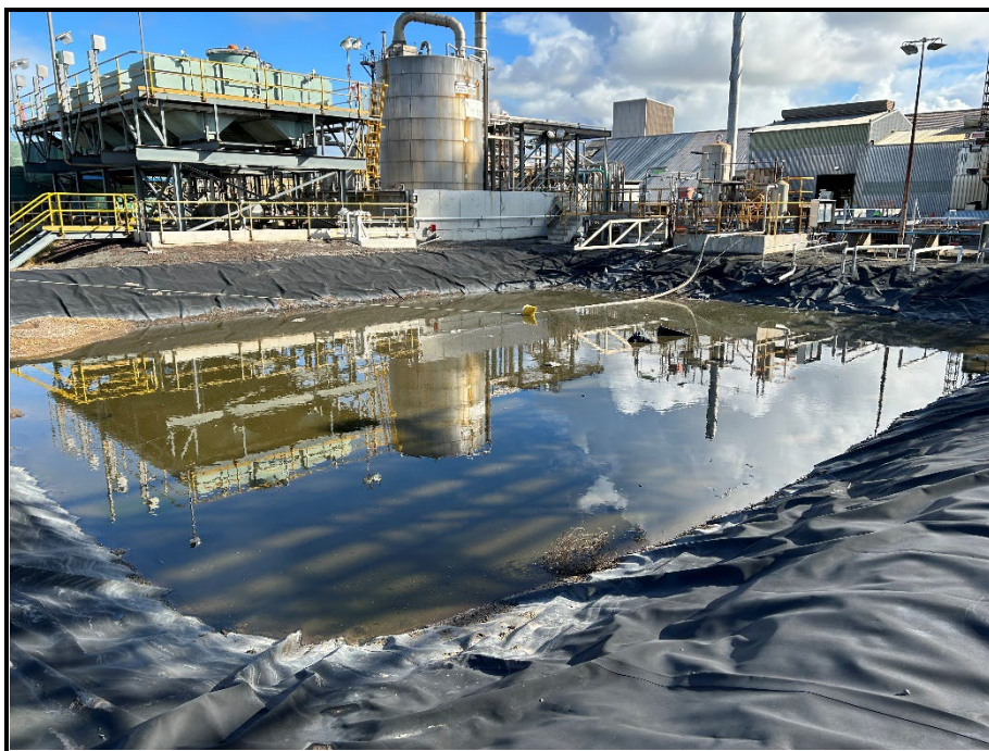
Photo 7: Effluent pond with single liner.
