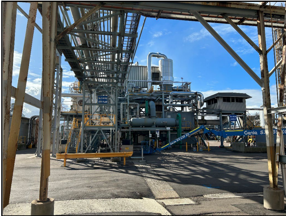
Photo 1: Nitric acid plant NAP3 with upgraded NOx abatement system.
