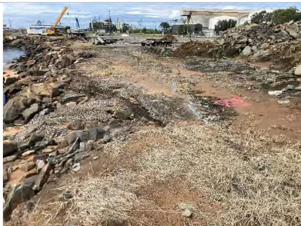
Photo 2-17 ACM observed across area immediately north of Site near BH08 (Chainage 70m to 100m)
