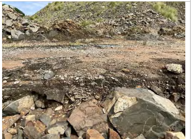
Photo 2-18 ACM observed within eroded embankment wall north of BH08 (Chainage 80m)
