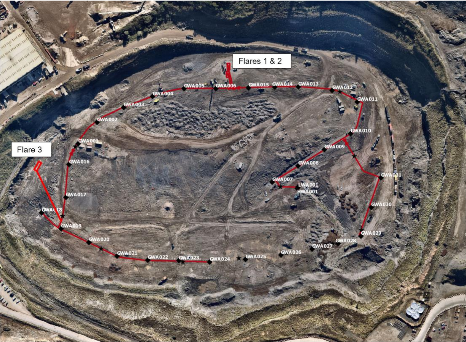
Figure 3: Preliminary LFG extraction system layout - As installed late June 2021 (Nearmap photo May 2021).
