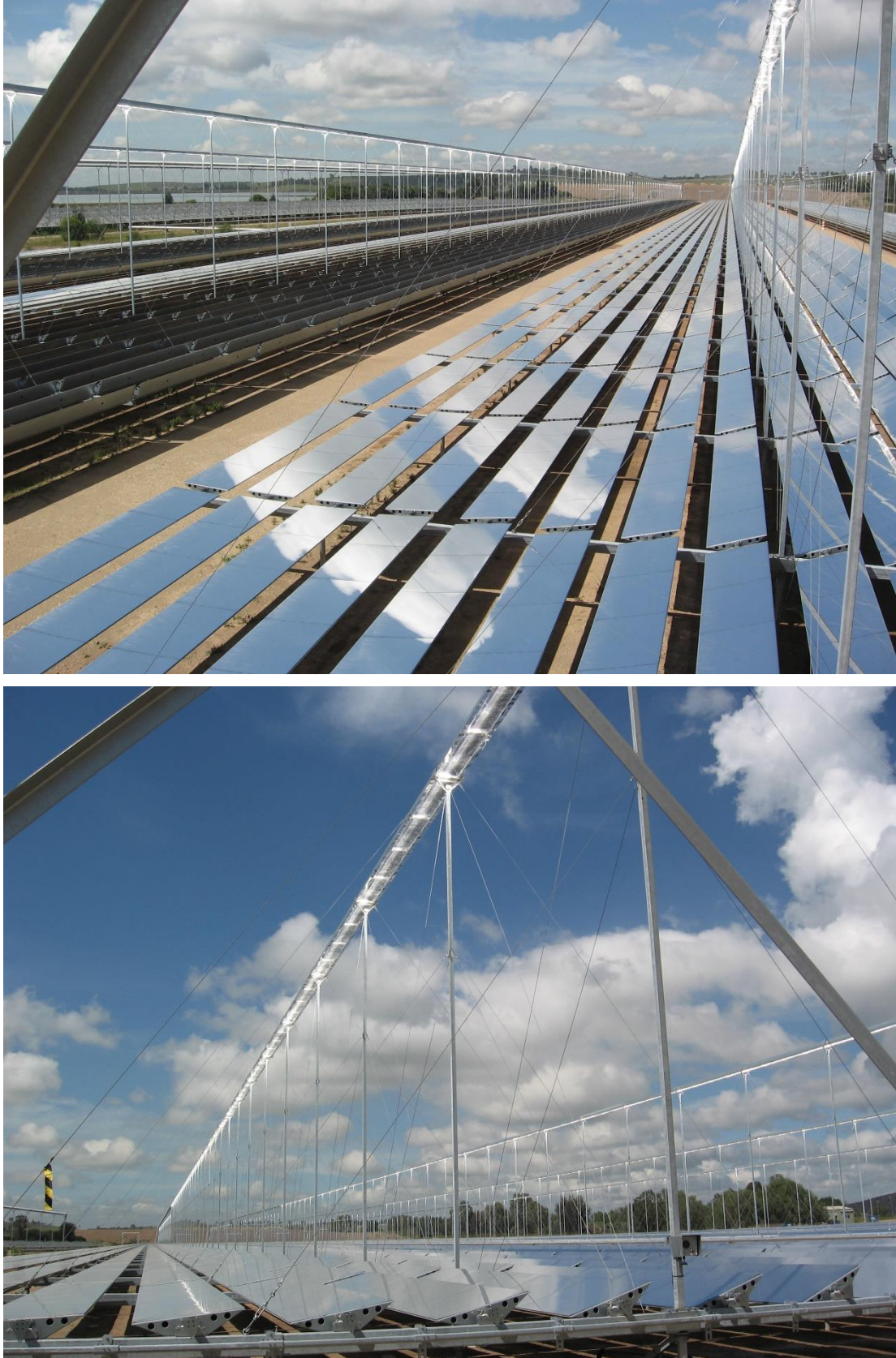
Figure 2 Existing solar array area
