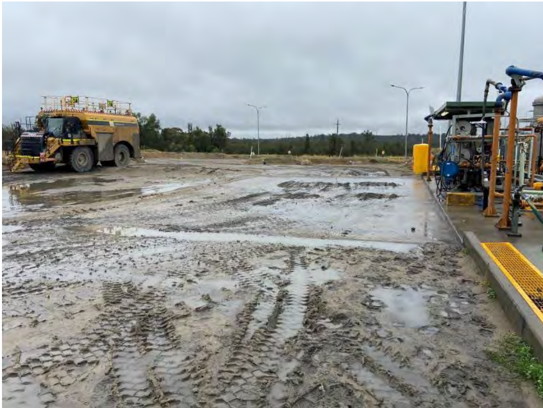
Plate 19 – Fuel fill up bunded area observed to have build-up of sediment during site inspection on 5 July 2022
