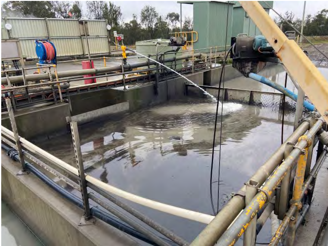
Plate 7 – Oily water separator near workshop during site inspection 5 July
