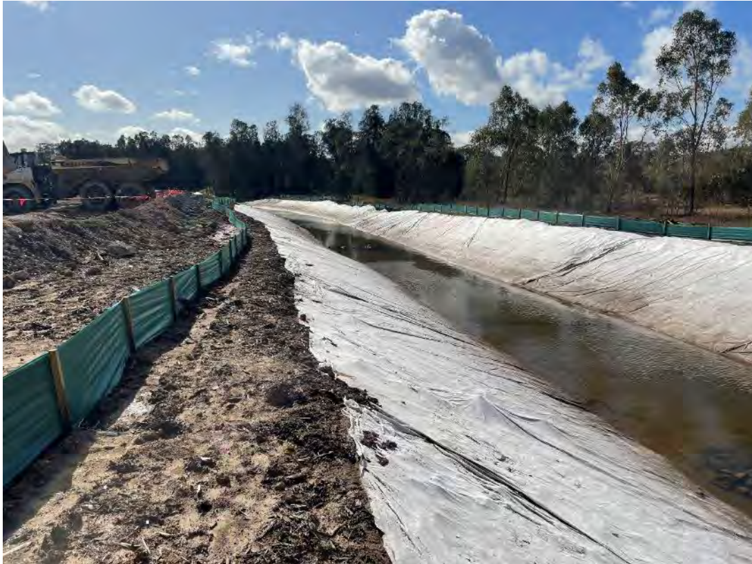
Plate 27 – Big Flat Creek Clean Water Diversion – Good example of Best Practice
