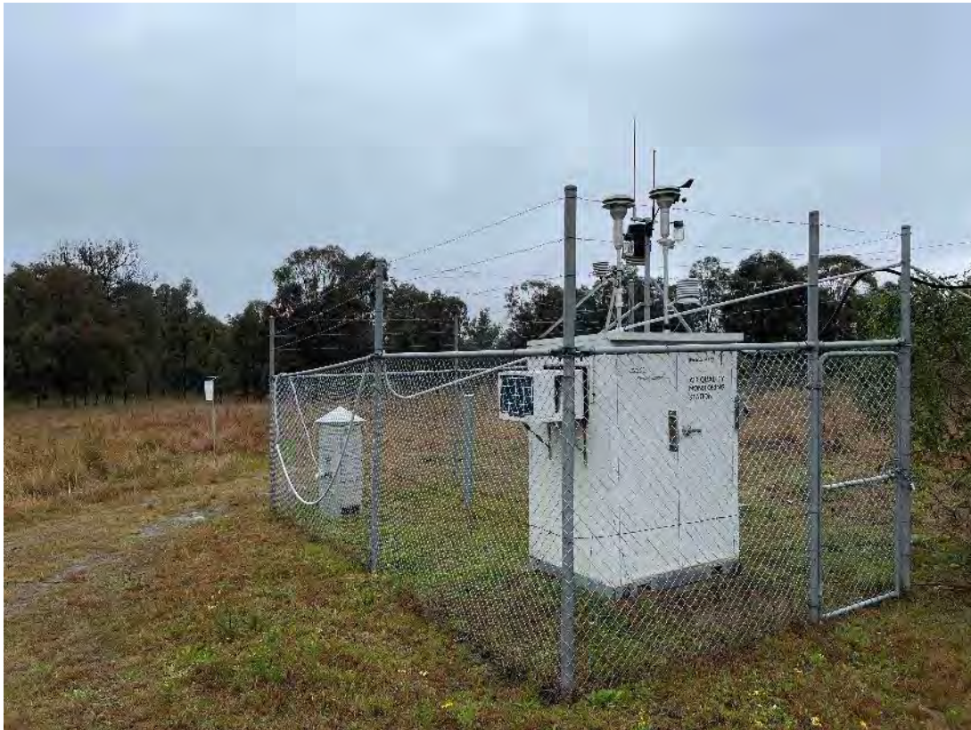
Plate 43 – Air quality monitoring station
