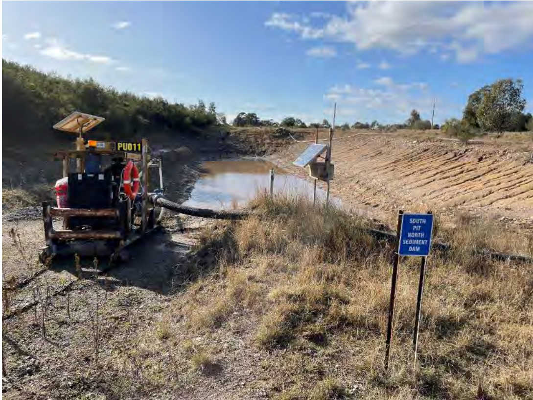
Plate 25 – South Pit North Sediment Dam – Same as the South Dam. Batters need to be rehabilitated.
