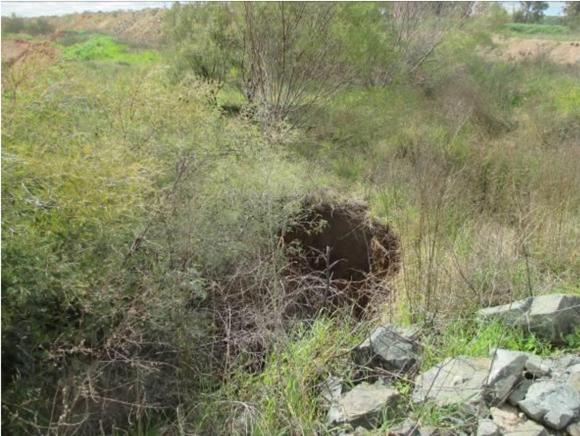
Figure 5: Wyoming 1 Open Cut looking north. Image displays a large gully with vertical sides and headcut.
