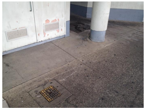
Figure 4.10: Example of subsurface services on the western side of Harbourside Shopping Centre
