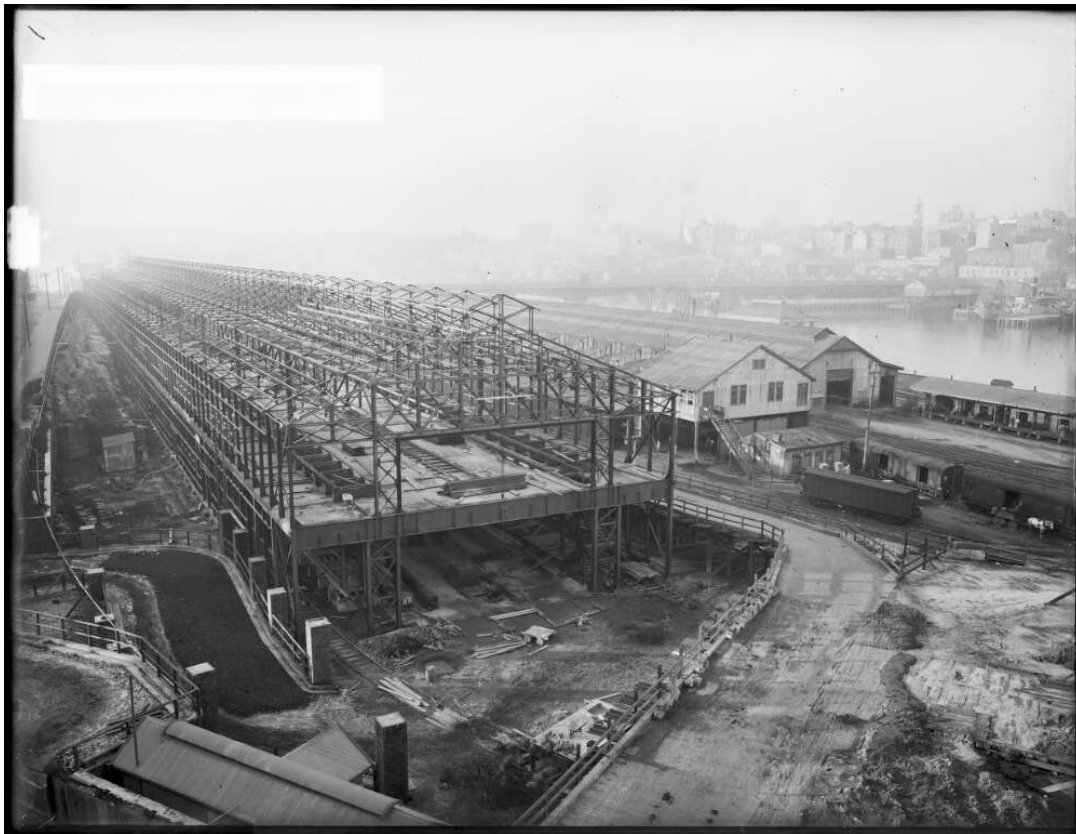
FIGURE 14: FRAME WORK OF DARLING HARBOUR SHEDS CONSTRUCTION, NEW SOUTH WALES (C1920). IMAGE SHOWS THE 1902 OUTWARDS GOODS SHED A&B AT THE RIGHT, THE 1891 SHED C&D IN THE CENTRE AND THE 1823 DOUBLE TIER SHED AT THE LEFT UNDER CONSTRUCTION. SOURCE: NLA PIC P860/325 LOC COLD STORE PIC AGF
