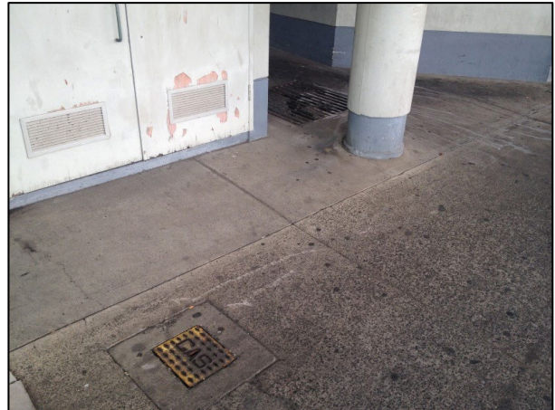
FIGURE 26: EXAMPLE OF SUBSURFACE SERVICES ON THE WESTERN SIDE OF HARBOURSIDE SHOPPING CENTRE.
