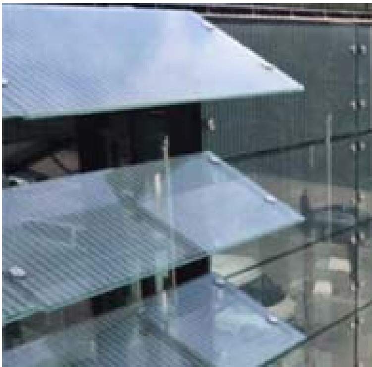
GLASS VENTILATION LOUVRES (LV1)
