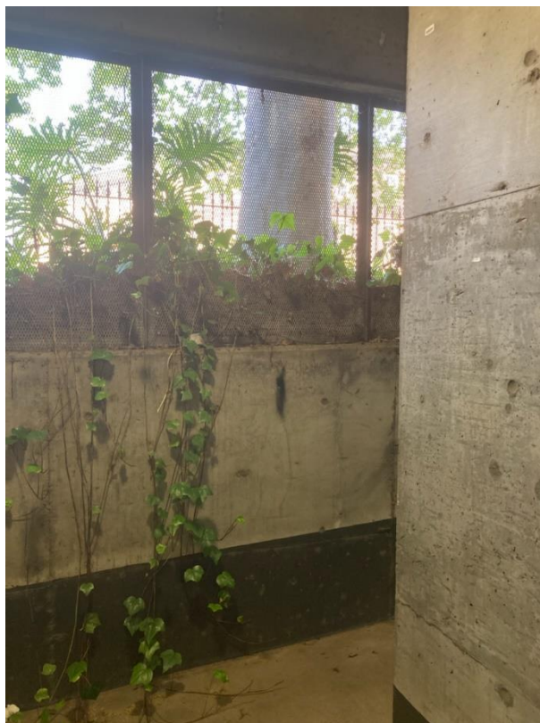
Tree 51: structural crack to retaining wall (top to bottom) at centreline of tree trunk
