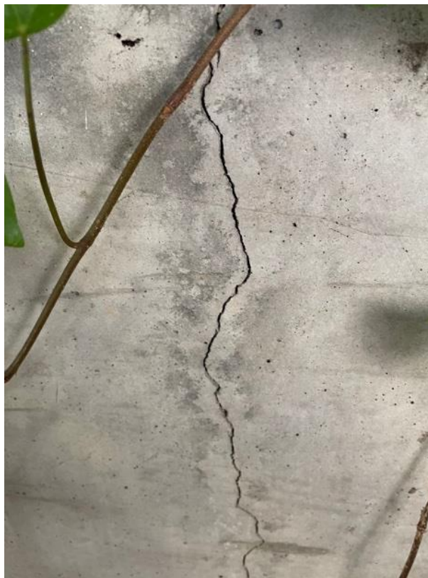
Tree 51: structural crack to retaining wall
