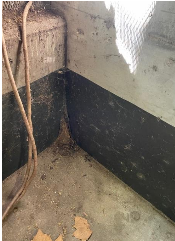
Tree 50: Plane Tree root penetration at wall floor internal junction
