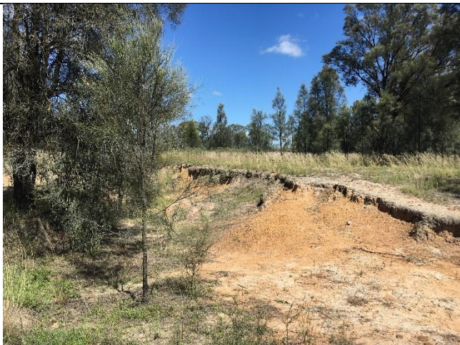
Photo 5 – LID3 erosion monitoring
