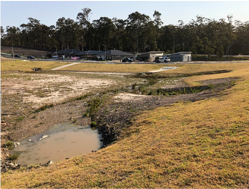
Figure 6.1: Retention basin located downstream of the DMA site
