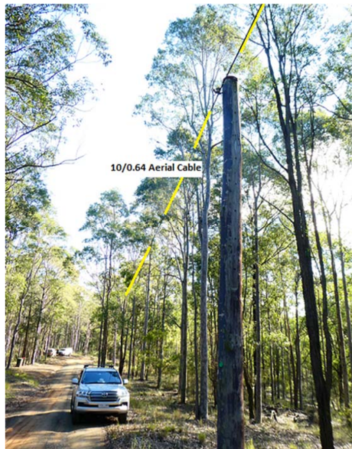
Figure 2 – View along Binalong Way showing 10/0.64 area cable mounted on Telstra poles
