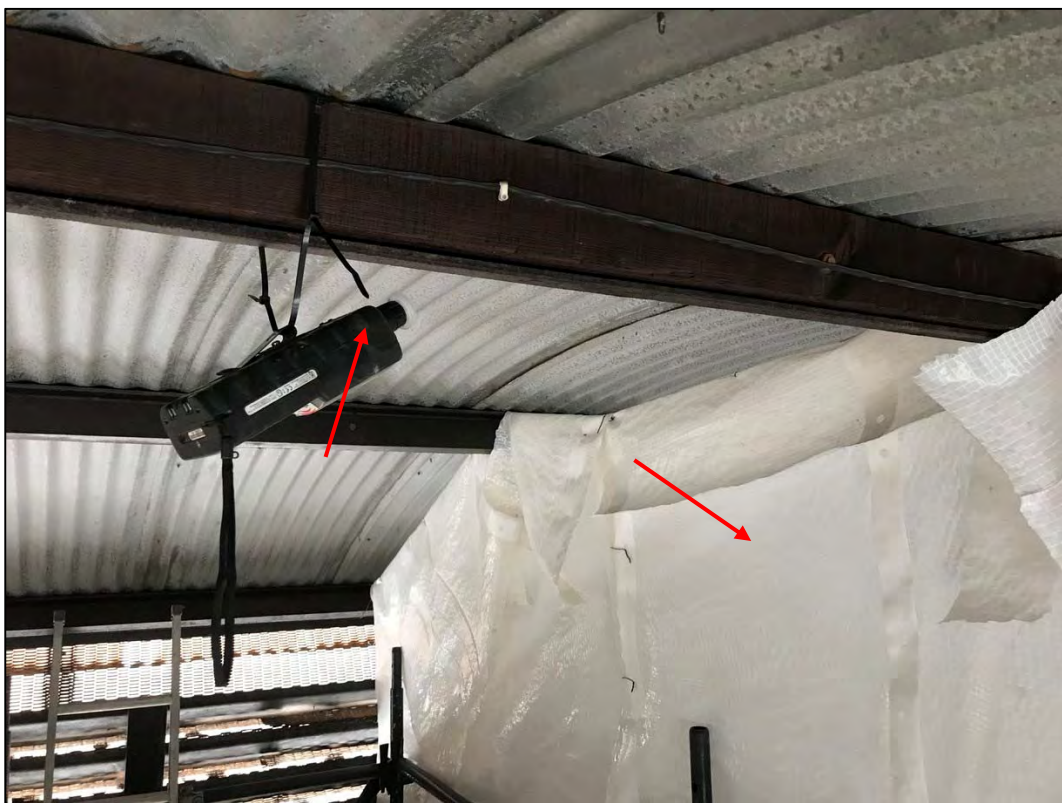
Photograph 6: Additional carbon monoxide monitoring following construction of the separation wall.
