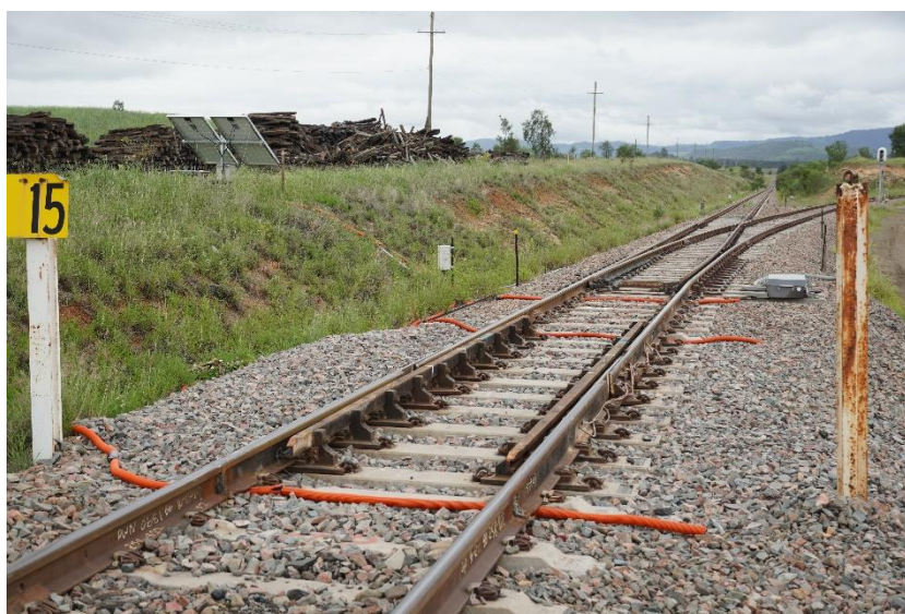
Figure 7-11 Rail expansion switch
