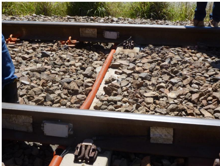
Figure 8-6 Track strain and temperature gauges
