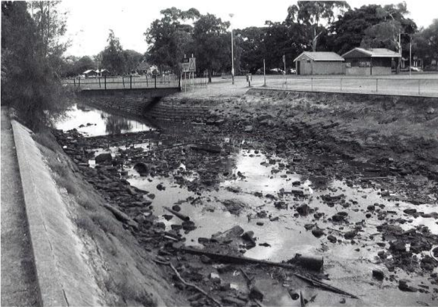
Figure 14. Sediment and base of Hawthorne Canal and merging point of old and new walls (Source: Sabolch, M., 2004. 'Sediment and rubbish at the base of Hawthorne Canal is visible at low tide.' In Sabolch, M., 2006. Hawthorne Canal , p. 97)
