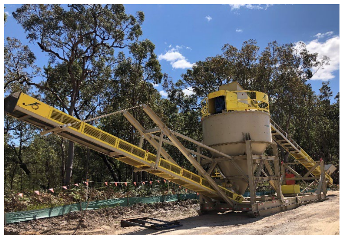
Photograph 2: Approved air separator onsite.
