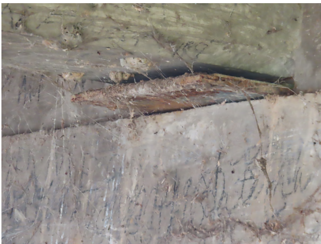
Photo 14. Tumbarumba (west) abutment. Centre beam bearing dislodged.
