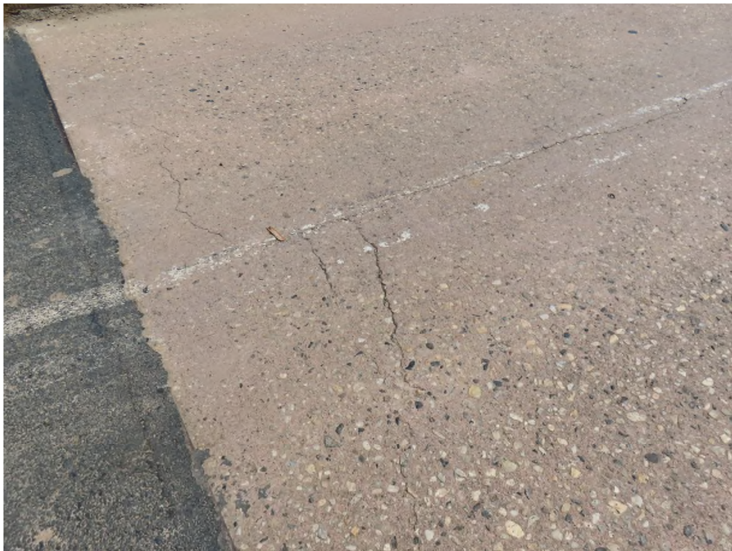
Photo 18. Transverse cracks in deck near east abutment.
