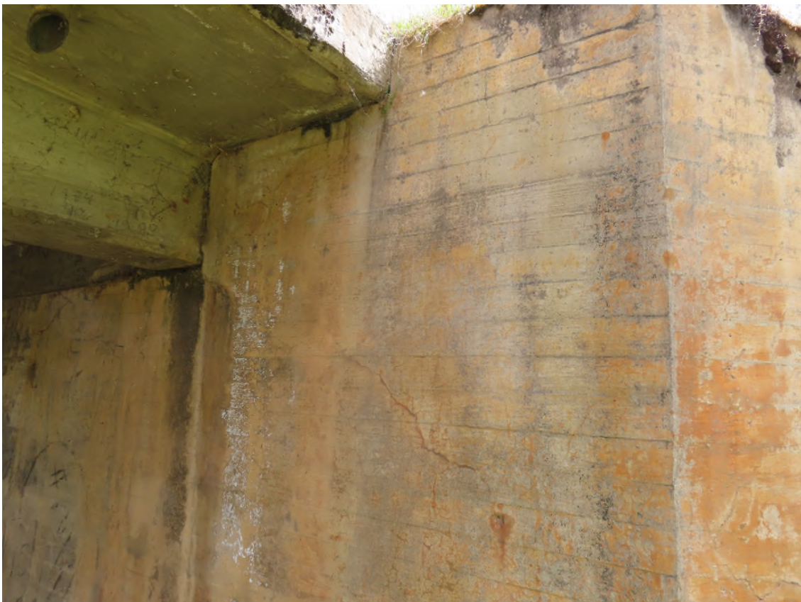
Photo 12. Typical crack in wingwall/abutment
