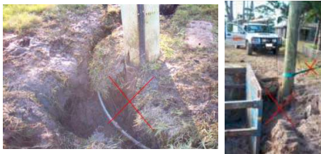
Above: Poles with become unstable if undermined
