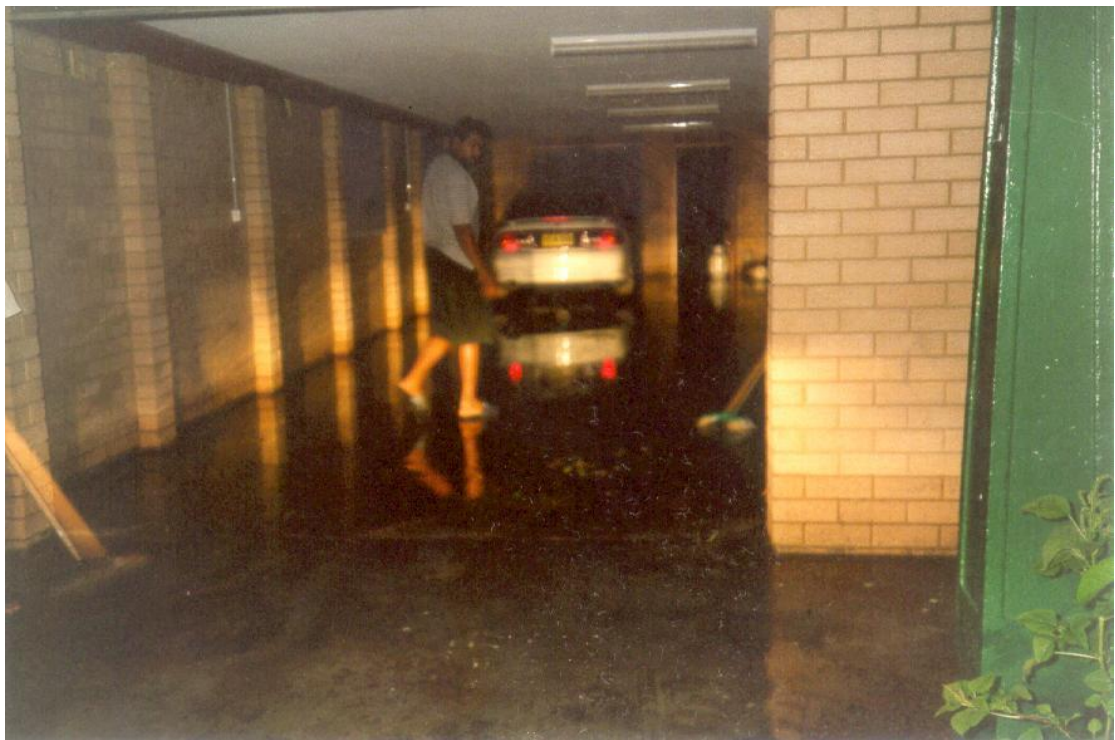
Aftermath of flooding through No. 62 Boronia Street, South Wentworthville following 16 February 2002 storm. Note tide marks present on internal and external walls indicating depths of inundation in the range 200 – 300 mm. [Finlaysons Creek Catchment]
