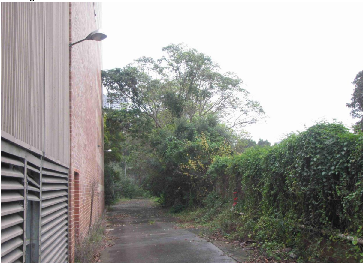
Figure 31 Shows again the brick retaining wall overgrown with English Ivy.
