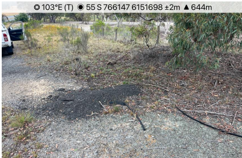
Photo 21: Bitumen with tyre tread and plastic on Hume Highway road shoulder near Lot 4 access gate (16/12/2025)
