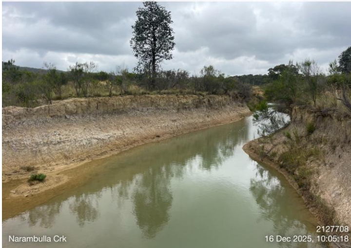
Photo 13: View looking south at steep and highly eroded creek banks of Narambulla Creek (16/12/2025)
