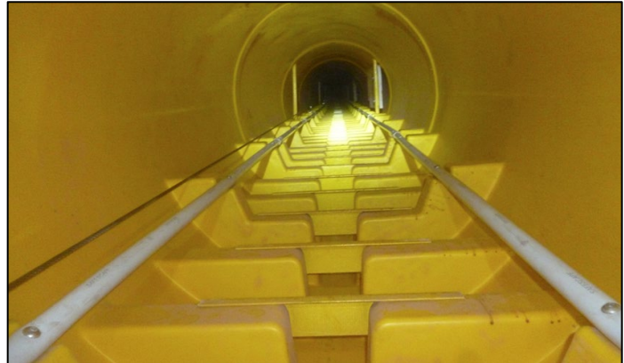
Figure 4: View inside a Safescape Ladder way
