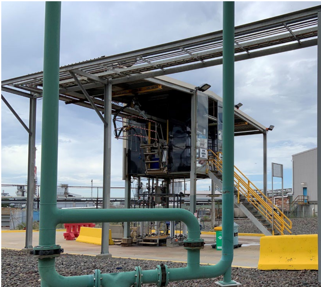
Figure 2.5 Existing sodium hypochlorite loading bay
