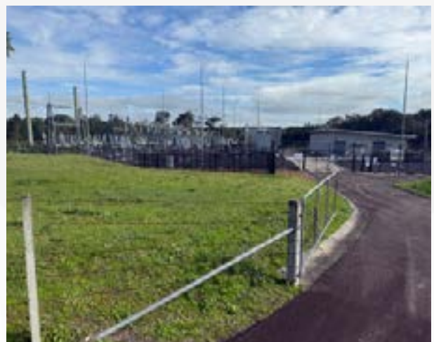
Photograph 6 Brandy Hill Substation
