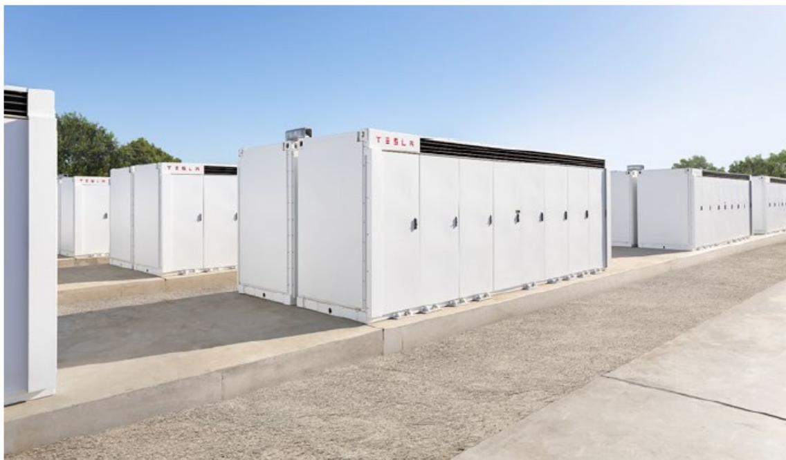
Figure 3-2: A typical BESS site
