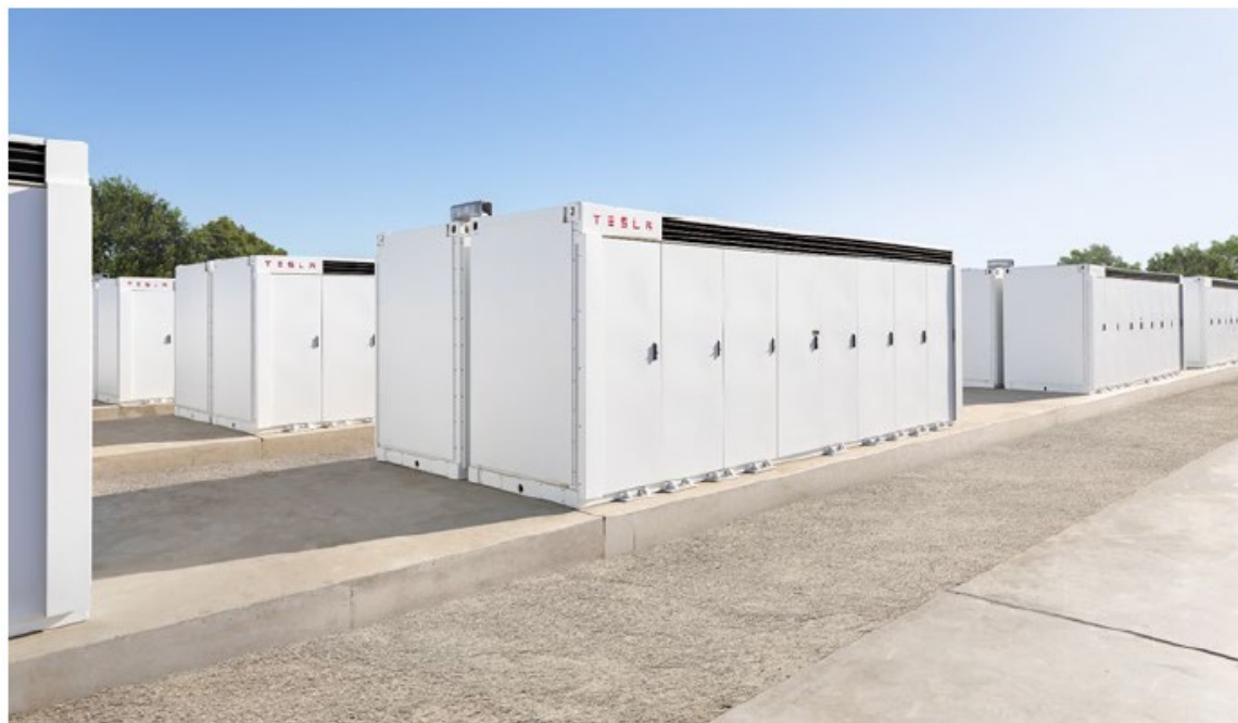
Figure 3-2: Typical multiple battery units
