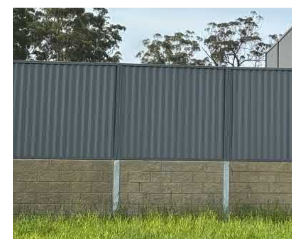
0.4 - 2.2m High Cantilevered Walls with Colorbond Fence RETAINING WALLS AND FENCES BETWEEN DWELLING SITES
