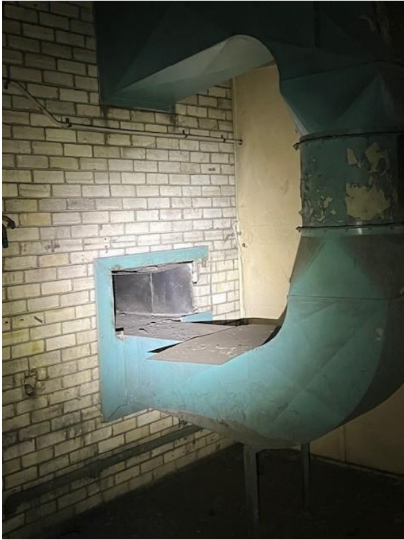
Photograph 19: Ventilation duct within dark room
