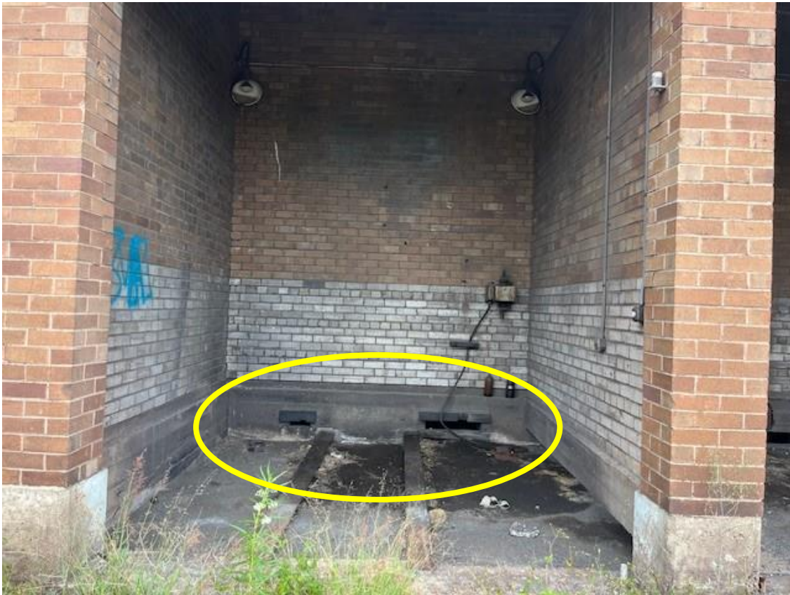
Photograph 15: Exterior of Roll Shop with entrance to confined space indicated by yellow circle.
