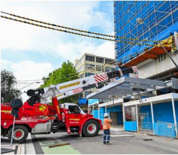
Figure 6 Installation of entrance awning at Clarke Street (Source: Sydney Metro, February 2024 Update)
