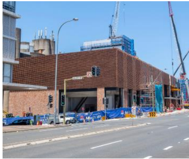
Figure 7 Completed brick façade work at Oxley Street and Pacific Highway (Source: Sydney Metro, February 2024 Update)
