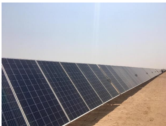
Figure 19- Mounted single axis bifacial tilting panels.
