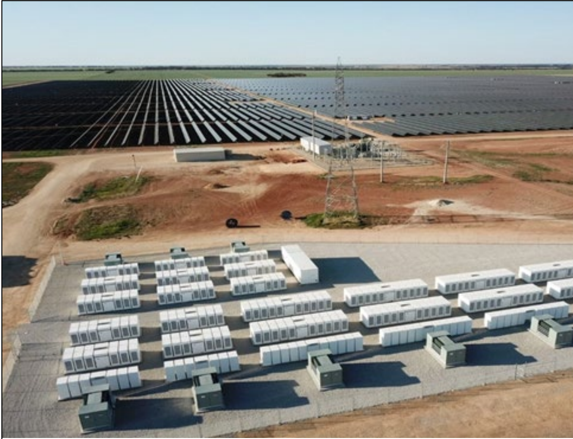
Figure 14: Example Battery Energy Storage System Design, Edify’s Gannawarra Solar Farm and Battery Project (Kerang, VIC)
