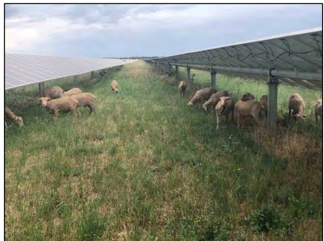
Plate 6: Edify Energy's Gannawarra Solar Farm (2020)
