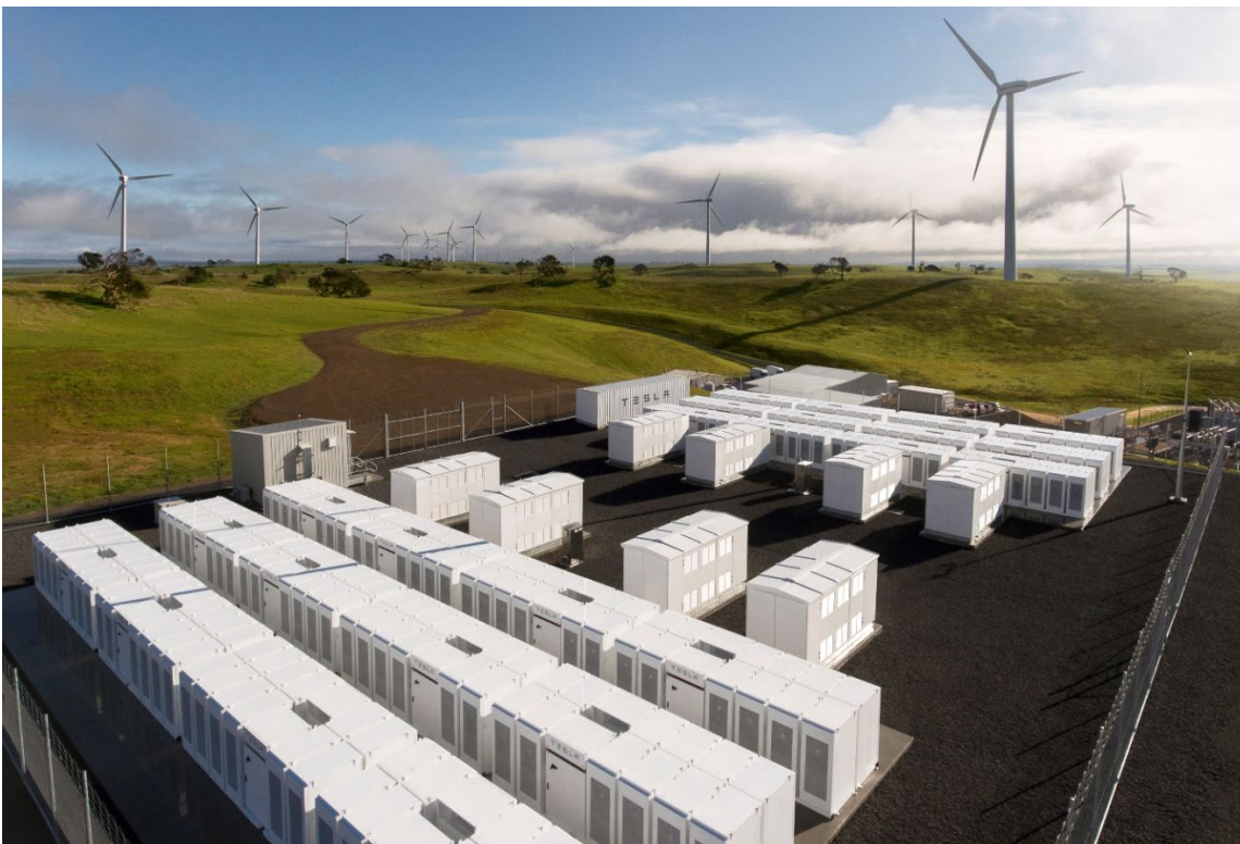
Figure 2-1 Lake Bonney Li-ion Battery Energy Storage System (Iberdrola)
