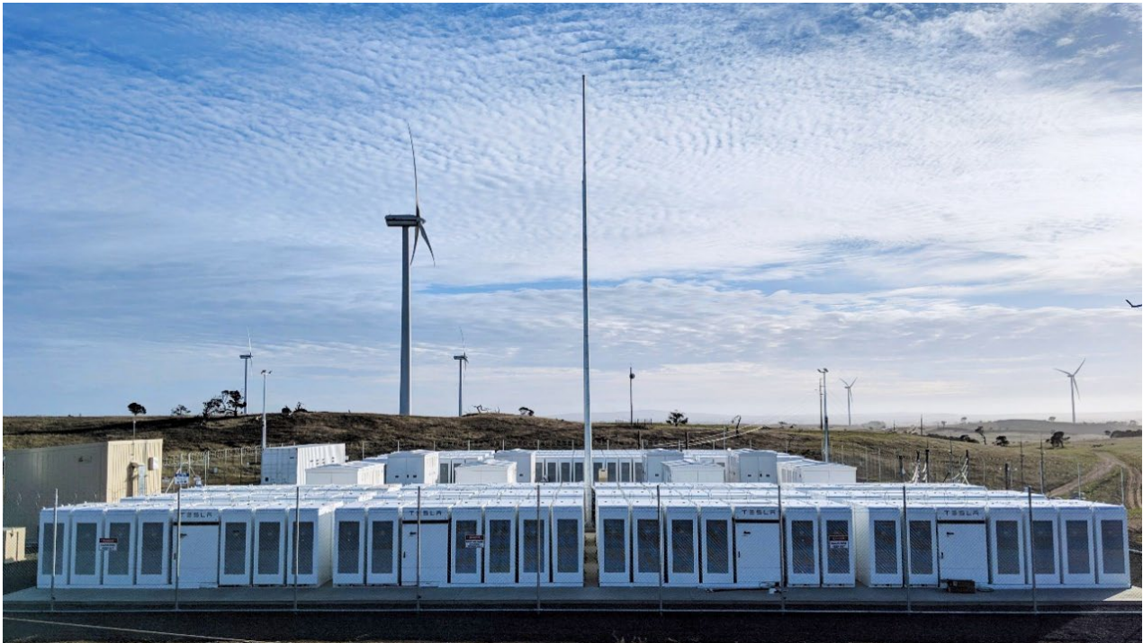
Figure 2 - Lake Bonney Battery in South Australia
