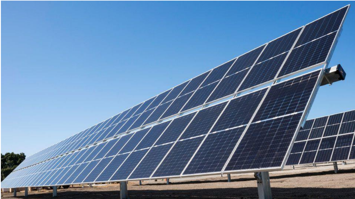
Photo 4-2: Example of a photovoltaic module (2P Configuration)
