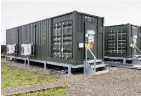
Plate 3-1a. Containerised battery example
