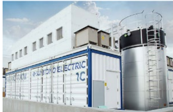
Plate 3-3b. Flow batteries (generally stacked)
