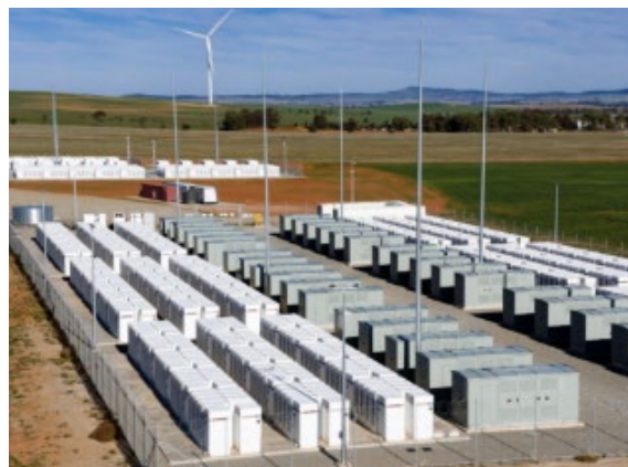
Plate 3-2c. Li-ion batteries (generally containerised)
