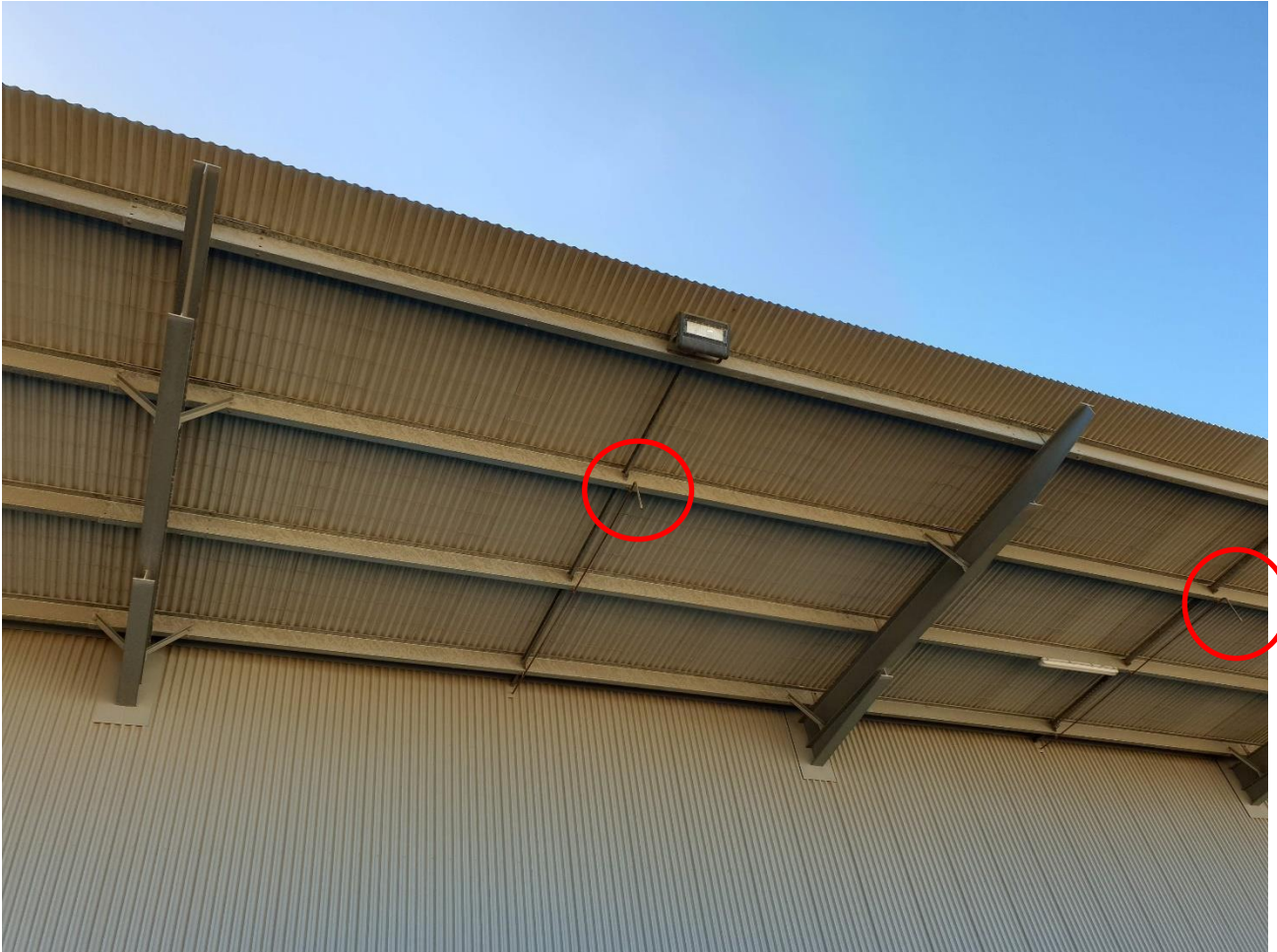
Photograph 2.6 Awning over storage bunkers – installed misting sprays circled
