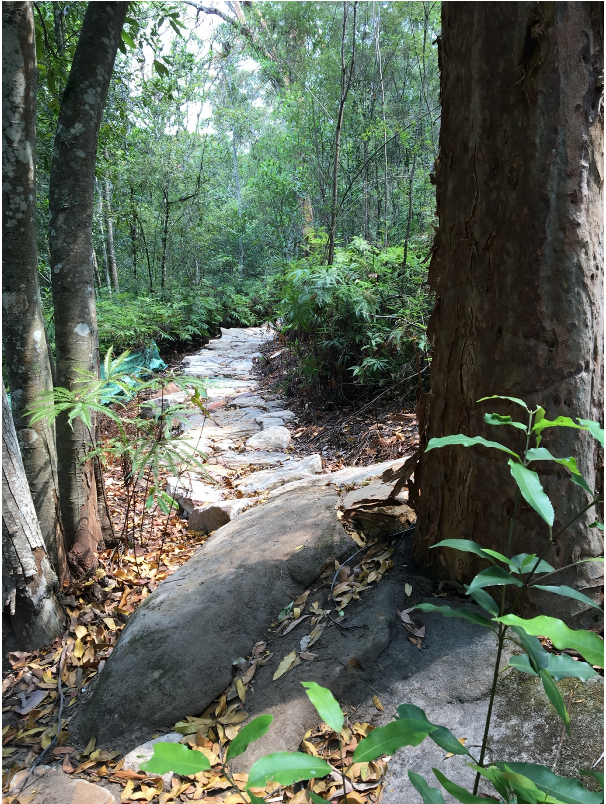
Figure 7 - Extensive rock armoring installed in a lower lying area of trail prone to flooding using imported sandstone (Location: Warimoo Downhill Track, Sydney NSW)
