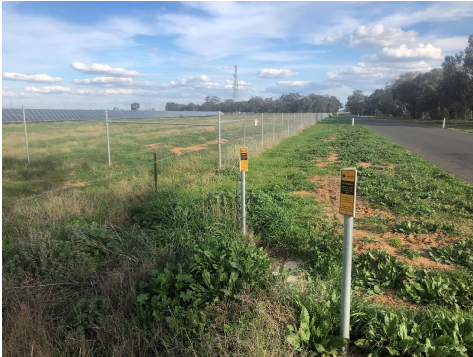
Figure 13 Darlington Point Solar Farm
