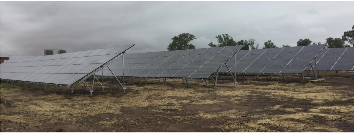
Figure 2-3: Example of Solar PV Panels
