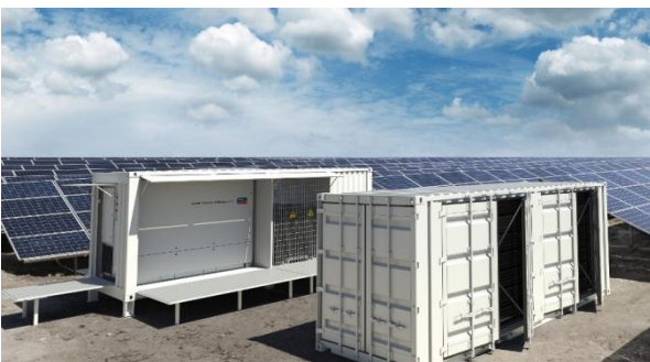
Figure 2-5: Example Inverter Kiosk
