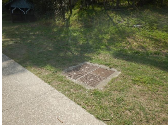
Figure 5.41: View northeast of utility vault
