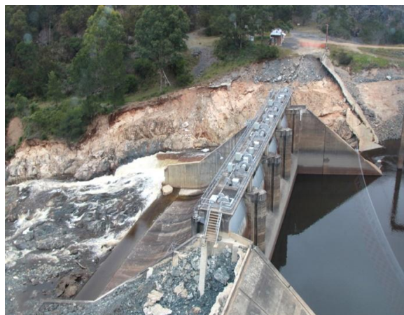
Oaky River Dam (post-failure), showing total collapse of the right embankment and damage to the left
