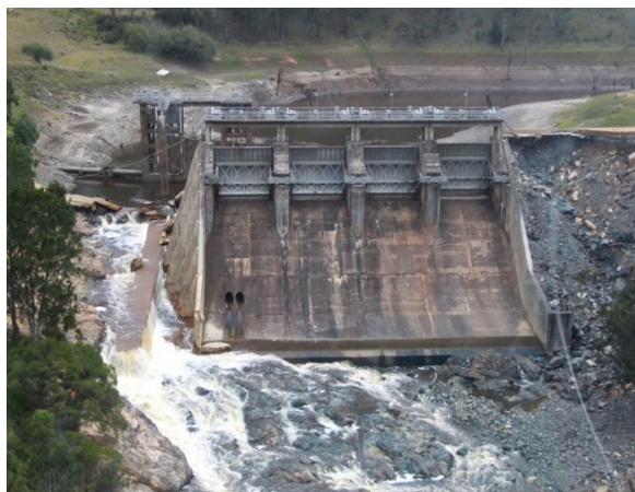
Existing Oaky River Dam (post-failure), looking upstream.
