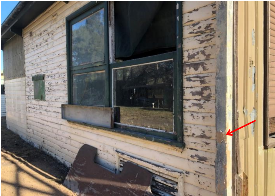
Photograph 29: Potting shed, external , downpipes, brown paint, lead paint (>0.1% lead w/w).
