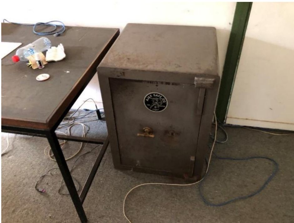
Photograph 42: Front Office, internal , "Ajax" brand safe, internal insulation, asbestos (assumed).
