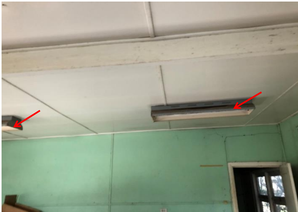
Photograph 61: Rear Office, internal , light fittings, capacitors, insulating oil, PCB (assumed).
