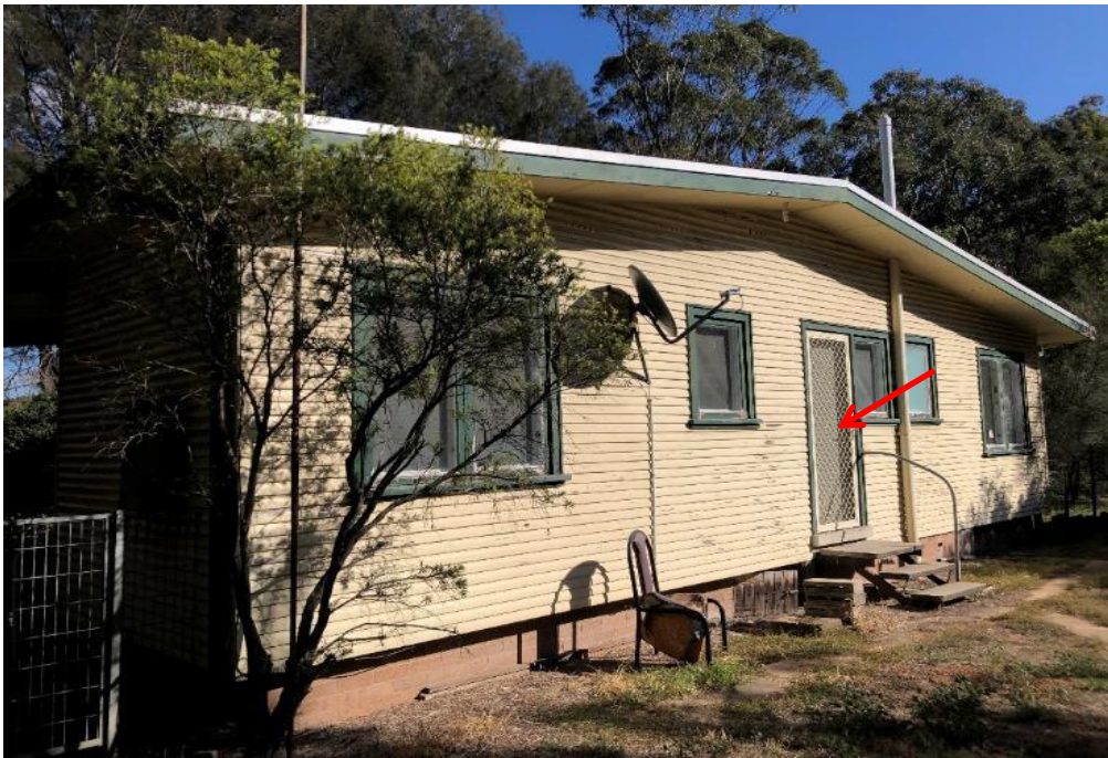
Photograph 13: Residential Dwelling, internal , laundry door, beige paint, lead paint (>0.1% lead w/w).
