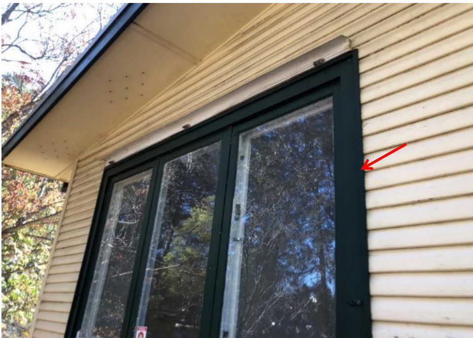
Photograph 8: Residential Dwelling, external , windows, green paint, lead paint (>0.1% lead w/w).
