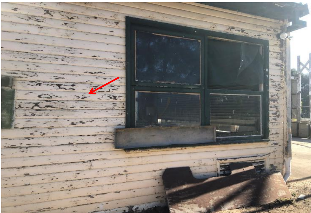
Photograph 22: Potting shed, external , walls, cream paint, lead paint (>0.1% lead w/w).
