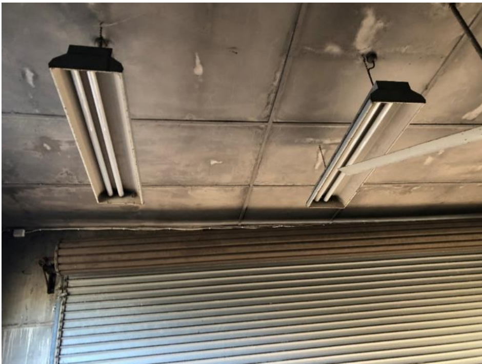
Photograph 30: Potting shed, internal , light fittings, capacitors, insulating oil, PCB (assumed).
