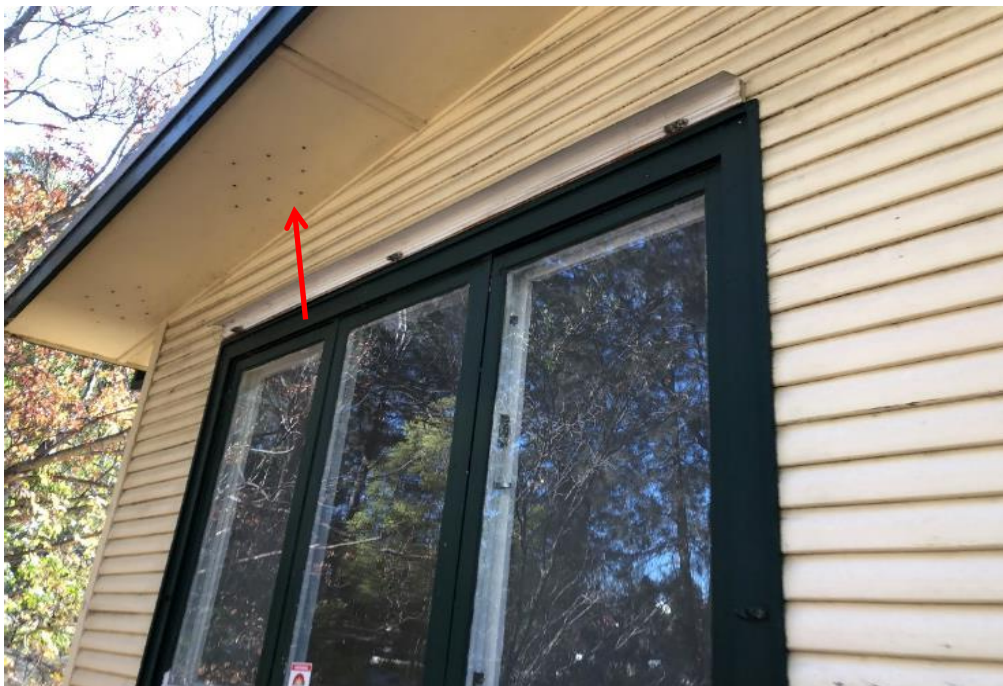
Photograph 5: Residential Dwelling, external, eaves, fibre cement sheet, asbestos detected by analysis.
