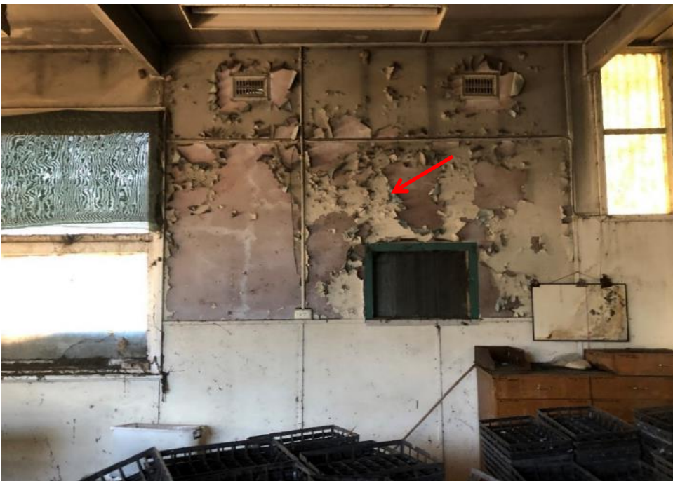
Photograph 32: Potting shed, internal , walls, beige paint, lead paint (>0.1% lead w/w).
