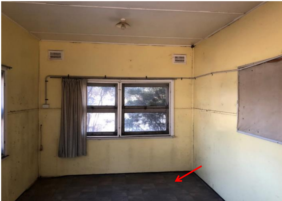
Photograph 54: Rear Office, internal , floors, vinyl floor sheet, no asbestos detected by analysis.
