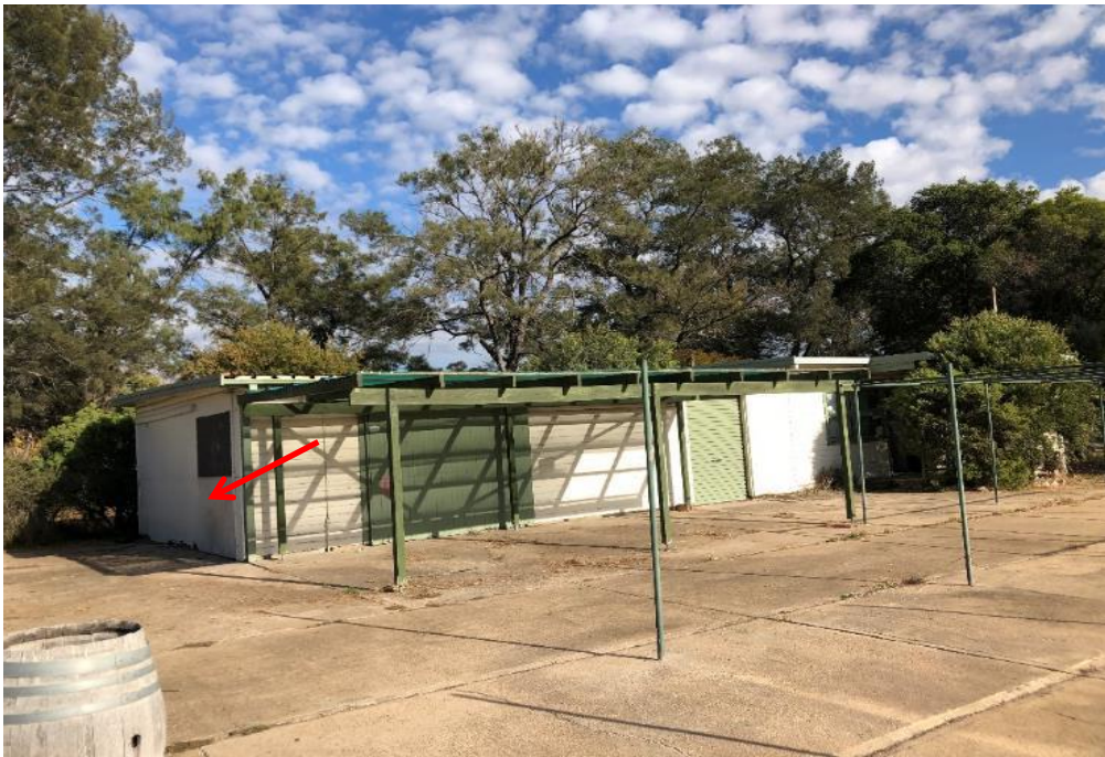
Photograph 36: Front Office, external, walls, south end, fibre cement sheet, no asbestos detected by analysis.
