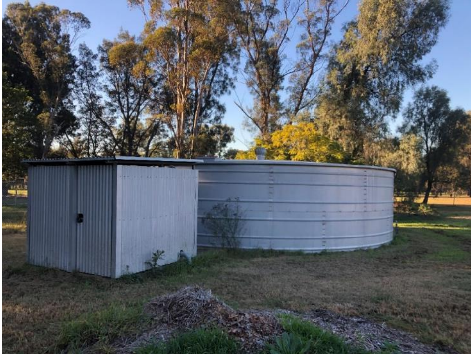
Photograph 19: Galvanised water tank.
