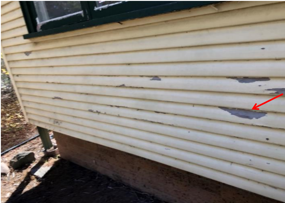
Photograph 7: Residential Dwelling, external , walls, beige paint, lead paint (assumed).
