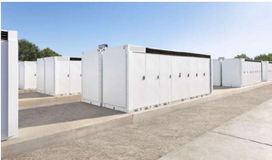
Figure 7: Typical BESS site
