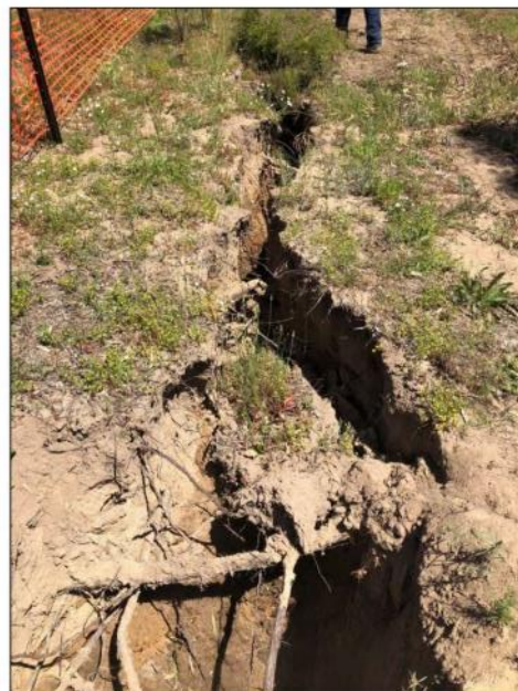
e) Wider crack near start line of longwall.
