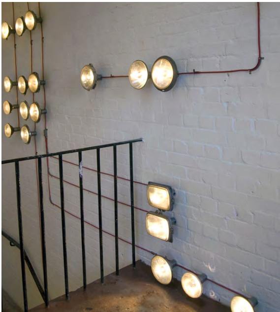
WALL MOUNTED LIGHTING
